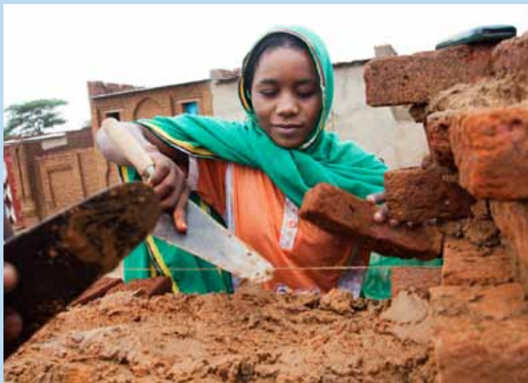
A young woman works on the construction of a community centre in Althoura Shemal in El Fasher, North Darfur, as part of a Community-Based Labour-Intensive Project (CLIP) sponsored by UNAMID DDR (Disarmament Demobilization and Reintegration Section), August 2012. (UNAMID/Albert Gonzalez Farran)
